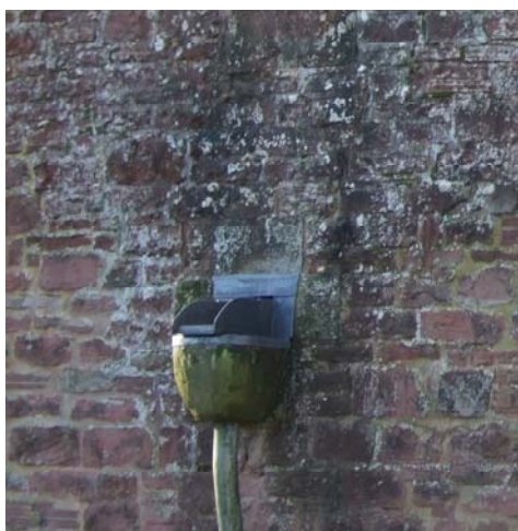
East wall hopper and overflow system
