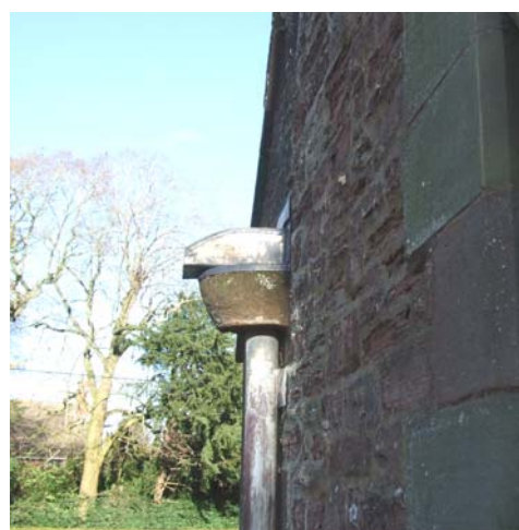
West wall hopper and overflow system
