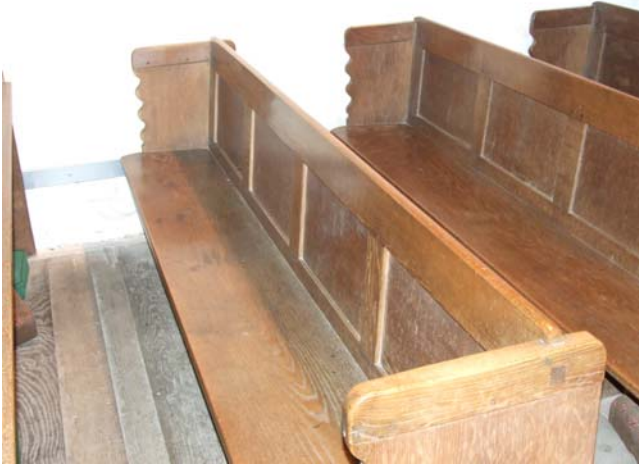
Front view of pews to show panelling, exposed tenon joint and wavy edge to the pew ends
