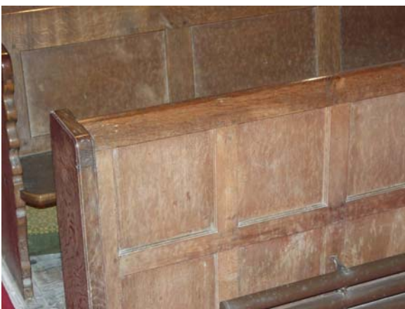
Front pew showing different style of panelling to that behind the seats
